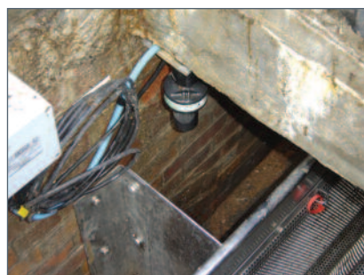
dB3 WITH DRIP SHIELD MOUNTED IN CSO CHAMBER
