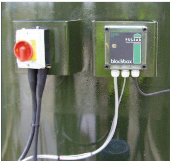
FOOD PROCESSING TANK LEVEL
