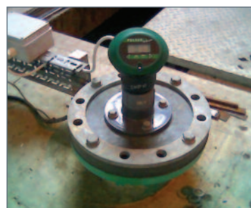
IMP ON A LIQUID LIME TANK
