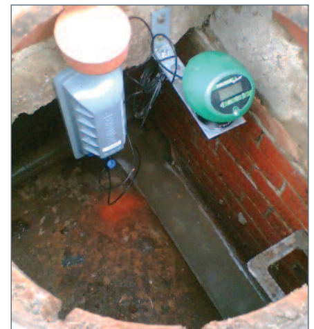
IMP MONITORING IN A CSO CHAMBER
